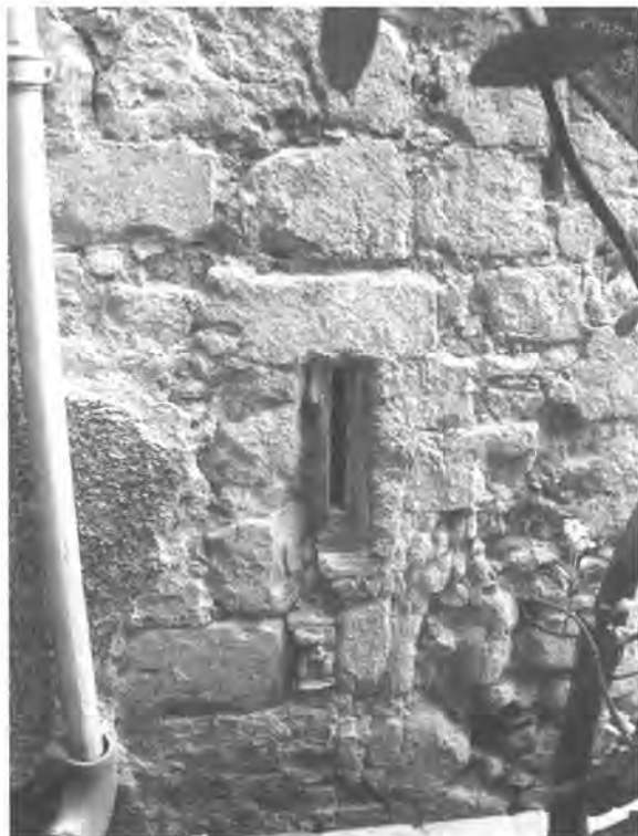
West face of the North Tower of the Gate House showing small window/arrowslit.
