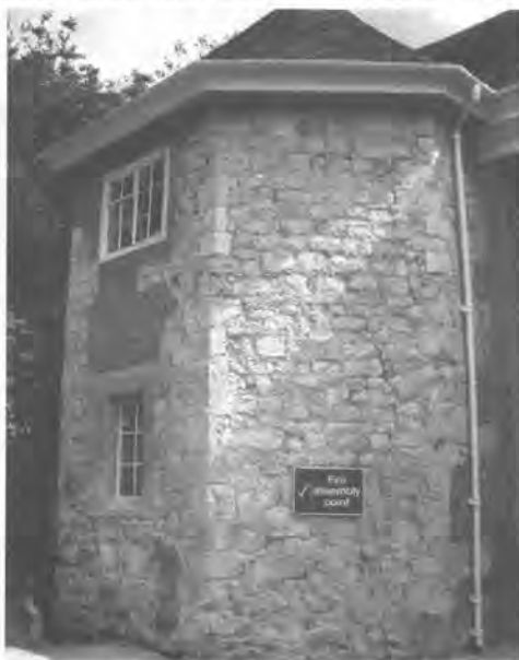
South-west face of the North Tower of the Gate House showing masonry coursing and crack running just to the right of the small notice.
